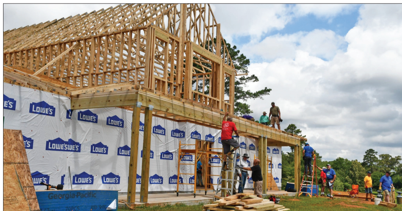
Staff Photo: Lucille Lannigan Volunteers with north Georgia nonprofit Builders for Christ construct the frame of a future foster family home in Calhoun County.
