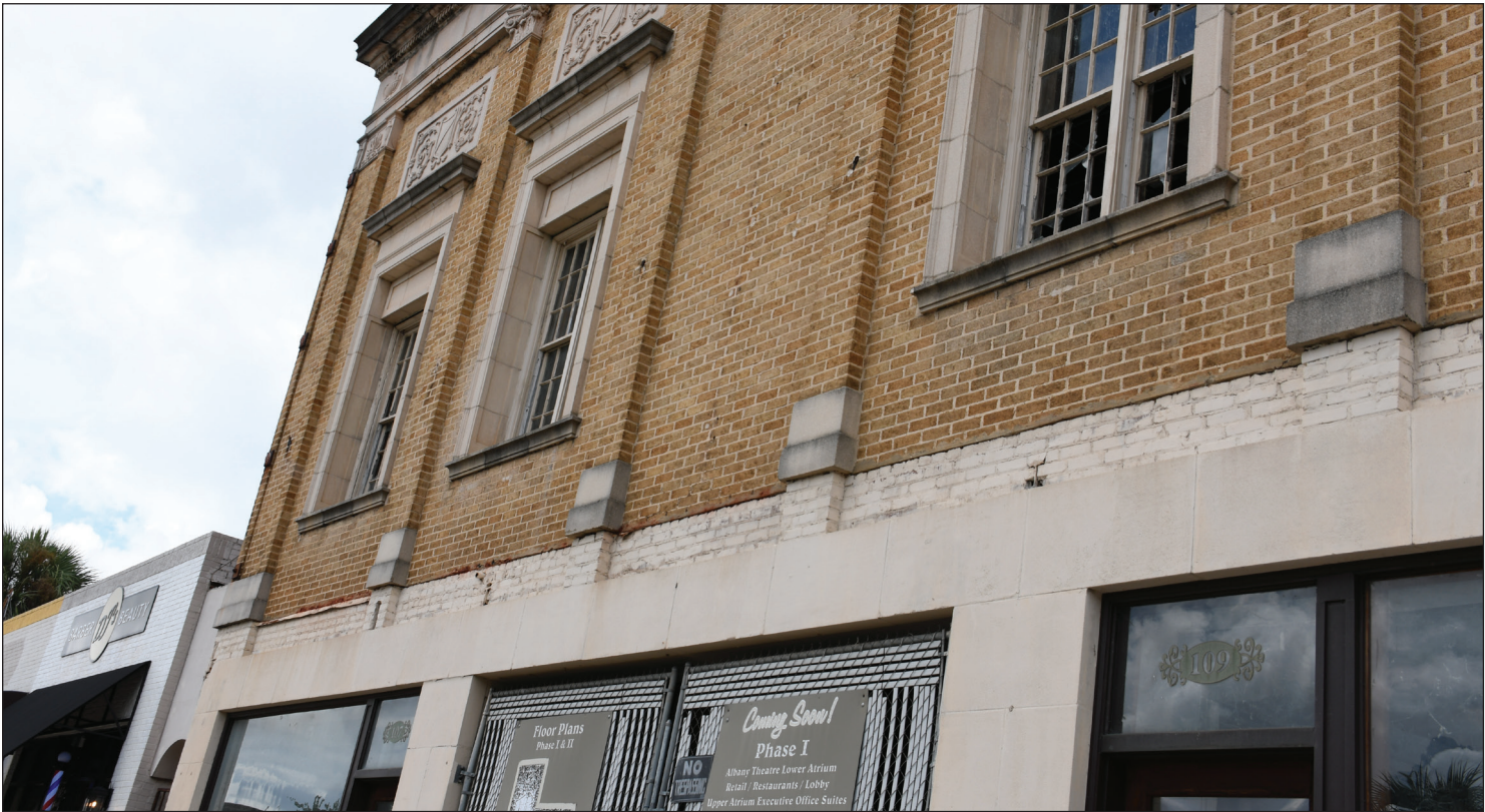
The Albany Theater building, which dates back to 1927, is one of two downtown theater buildings the city is seeking to preserve. The building was heavily damaged during a 2018 fire.
