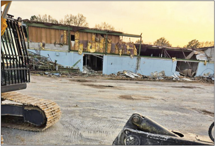
Special Photo The former Roses Discount Store and shopping center on East Oglethorpe Boulevard is being torn down 50 years after the center was constructed.
