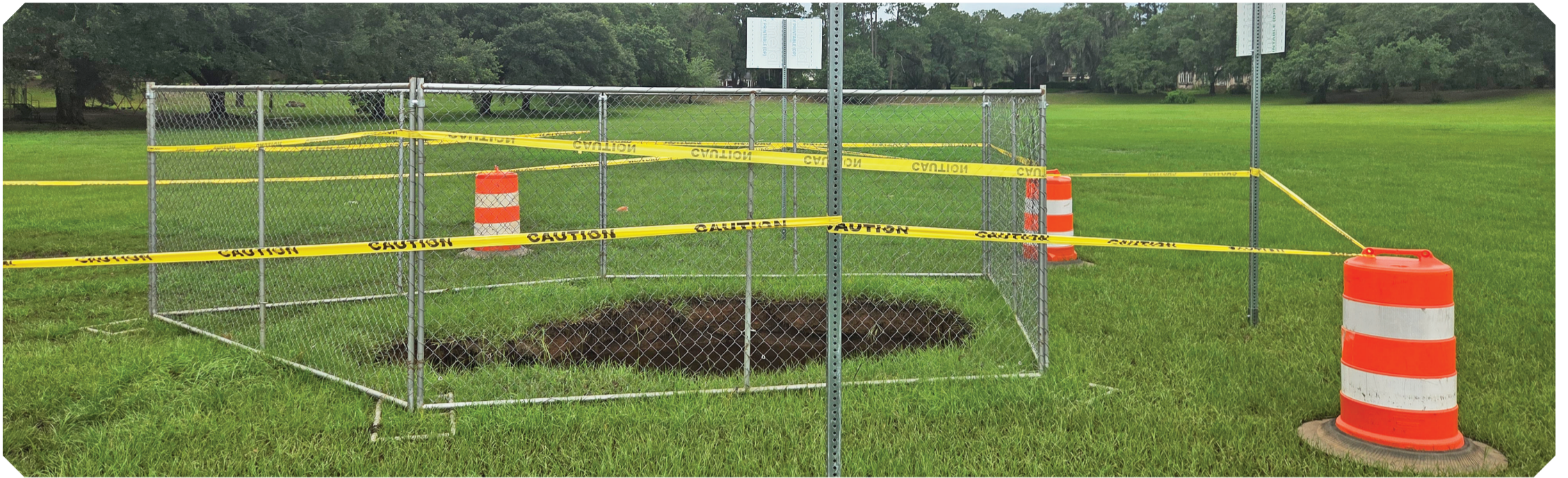
A sinkhole at Hilsman Park in Albany developed after recent heavy rains.
